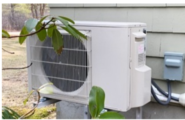
Outdoor heat pump unit, courtesy of Efficiency Maine
