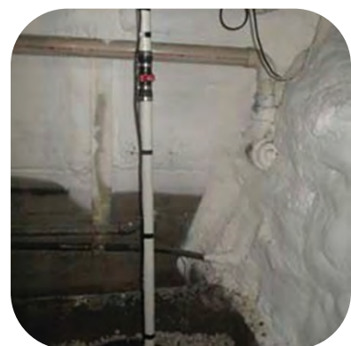
Sump Drainage with Check Valve
