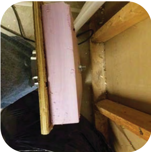
Build panels with maximum R-value allowed by cavity depth while keeping an air gap from exterior surfaces
