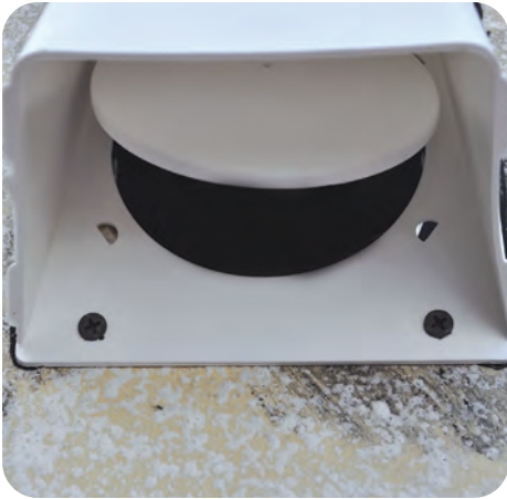
5. Termination has backdraft damper and no cage
